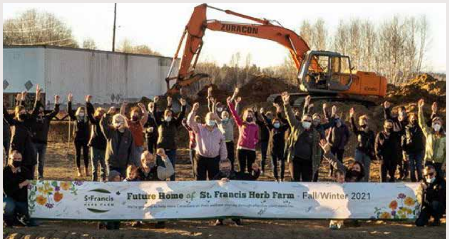
Members of the St. Francis Herb Farm team gather on site to celebrate the start of construction. PHOTO: COURTESY FACEBOOK/ST. FRANCIS HERB FARM
